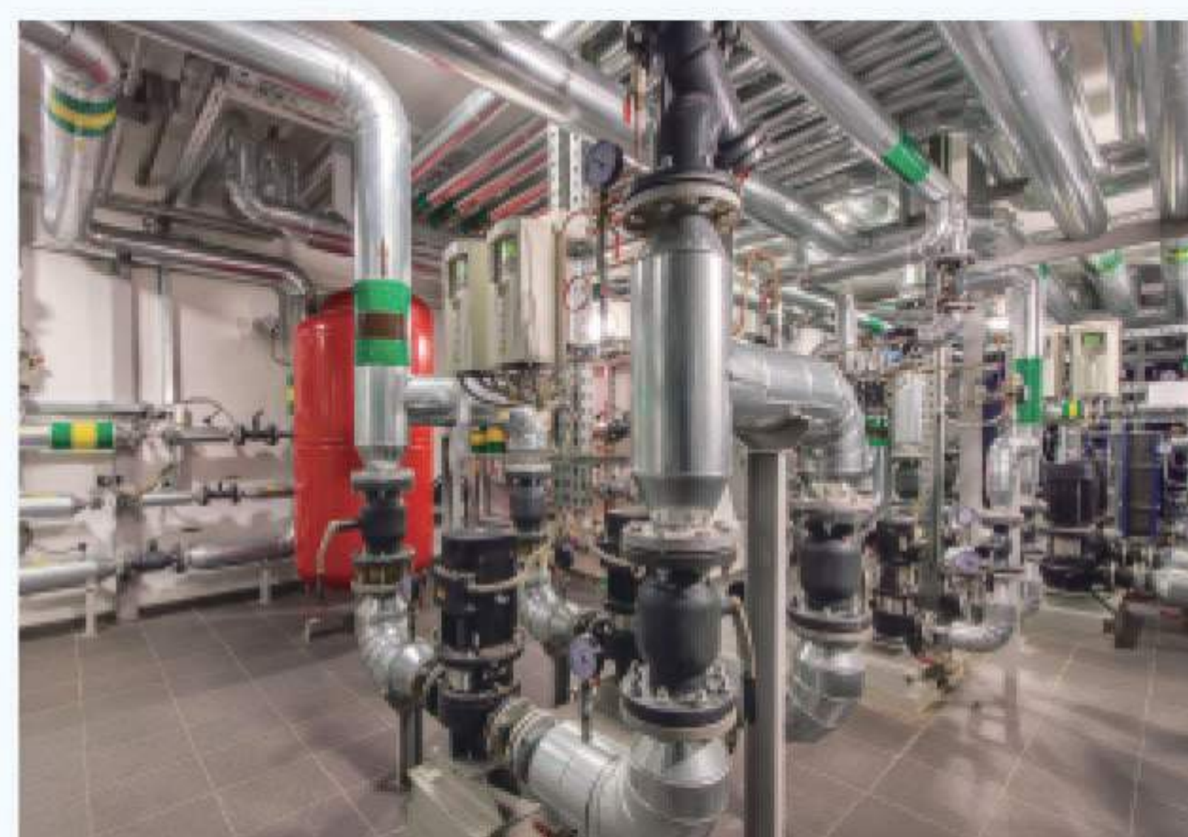
Municipal heating system
